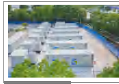
Zhejiang Xianhe New Energy ESS Project Scale: 44.72MWh
