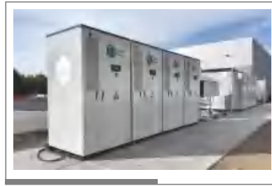
Belgium Distributed ESS Project Scale: 17.5MWh
