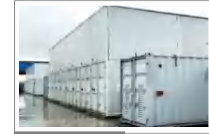
Jiangsu Shipyard ESS Project Scale: 100MWh
