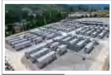
Yunnan Xiangyun Shared ESS Project Scale: 400MWh
