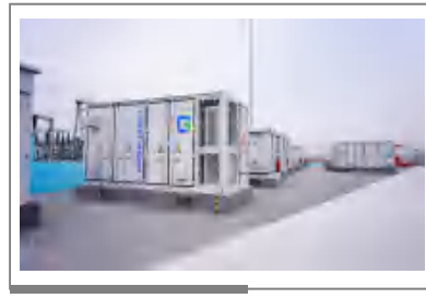
Anyang Shenlong Smart ESS Project Scale: 34.4MWh
