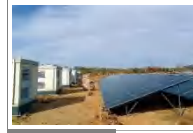
Germany Containerized ESS Project Scale: 16.77MWh
