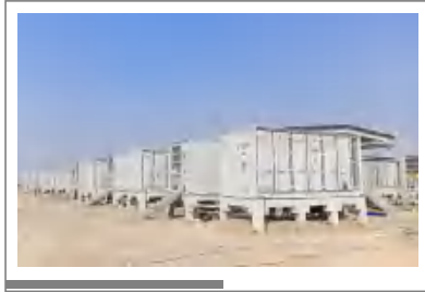
India ESS Project Scale: 722MWh(Total 1.5GWh)
