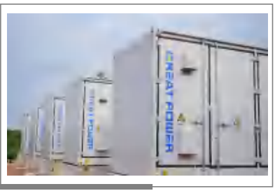
Hunan Anfu Environmental ESS Project Scale: 25MWh
