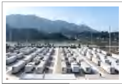
Sichuan Zhongfu Electrolytic Aluminum ESS Project Scale: 428.48MWh
