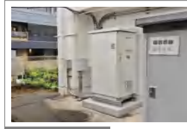
Japan, Yokohama School PV + ESS Project Scale: 17.5MWh
