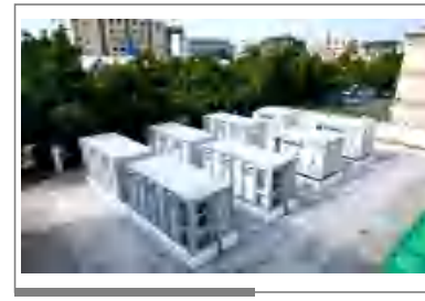
Zhongshan Zhongjing Semiconductor Smart ESS Project Scale: 27.52MWh
